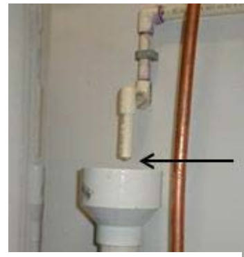
Air gap in softener backwash drain line
