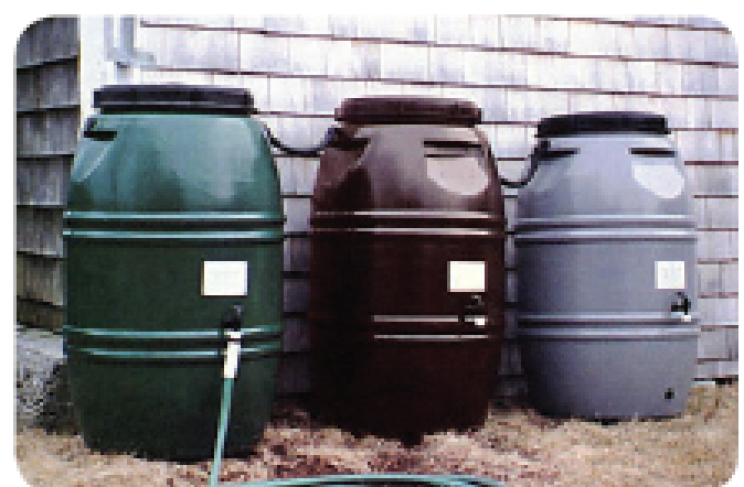
Runoff-reducing rain barrels
